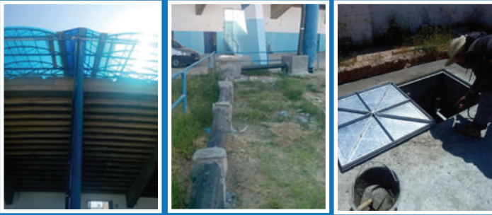
Rain Water Harvesting Pilot Project for the stadium
