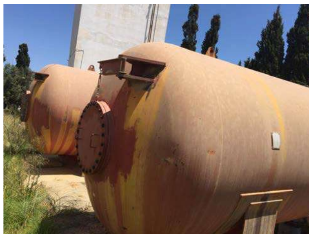
Figure 23: The existing surge vessels in the Monastir pumping station
