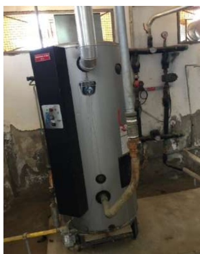
Figure 6: Stadium gas boiler
