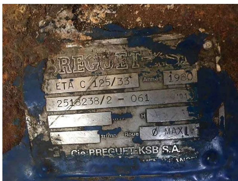
Figure 21: Pump Name Plate
