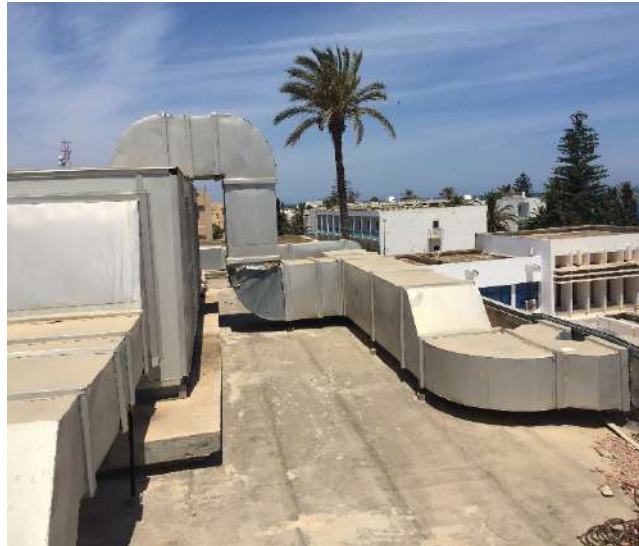
Figure 3: VRF system from the site
