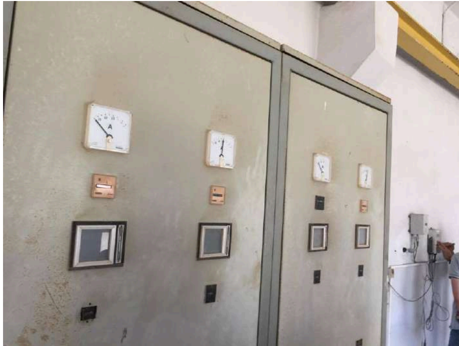
Figure 22: The existing flow meter (right) and the electricity sub-meters in the pumping station
