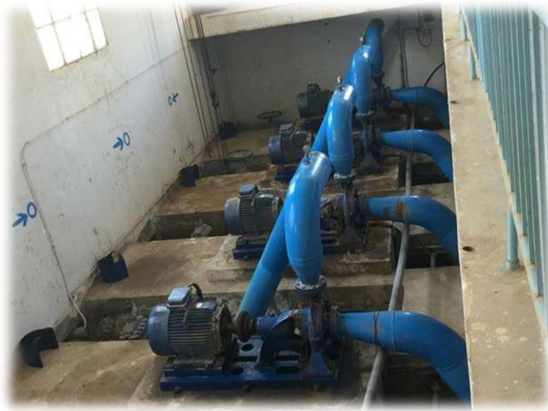
Figure 138: Water supply pumps as assembled with components
