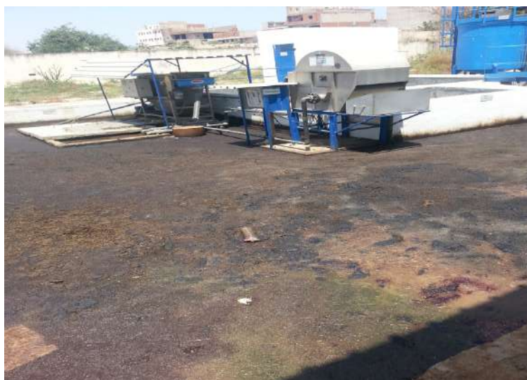
Figure 16: Bio-waste treatment unit
